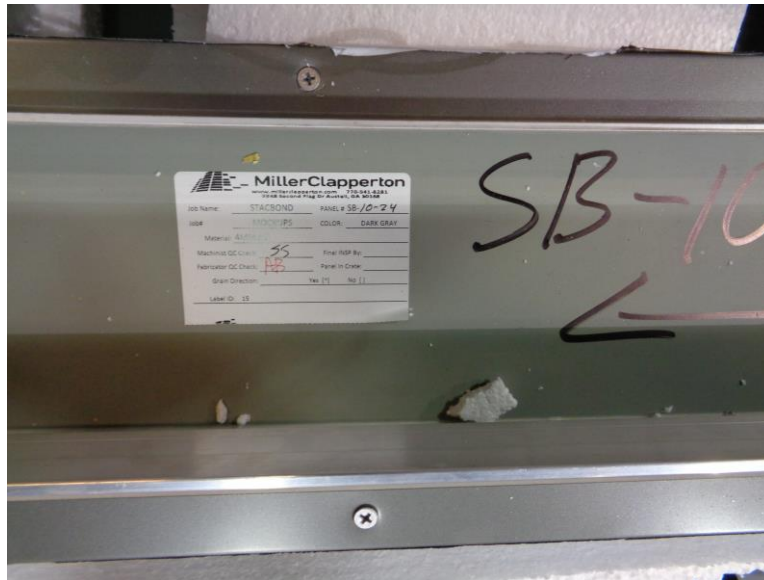
Photo No. 3 Panel Labeling
