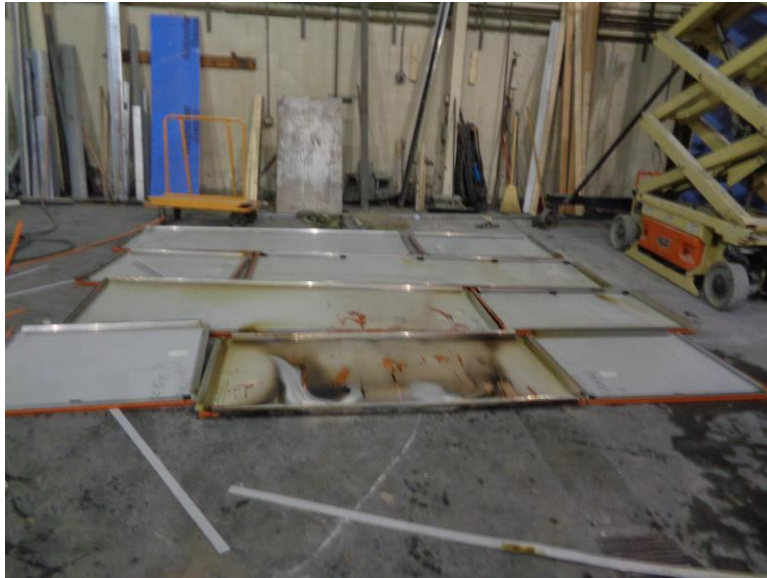
Photo No. 13 Back of Panels
